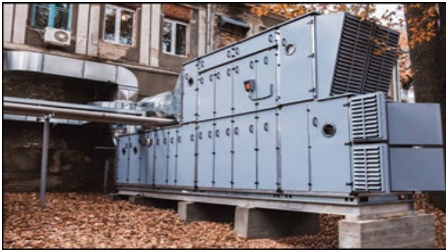
Figure 10. Commercial Air Handling Unit
