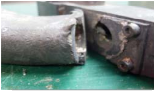
Figure 10. Broken pump (Platform A)
